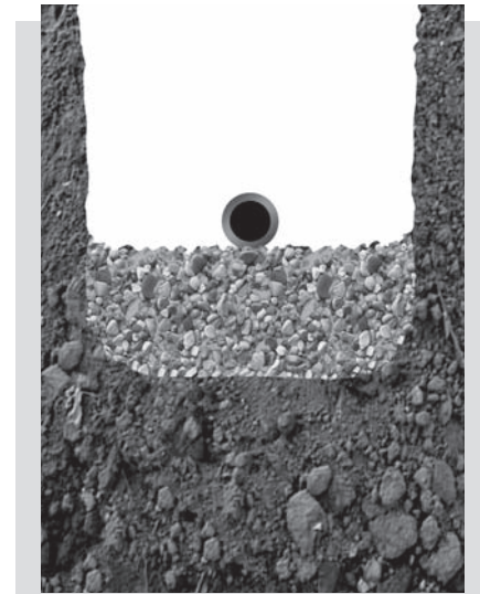
Trench in poor soil
