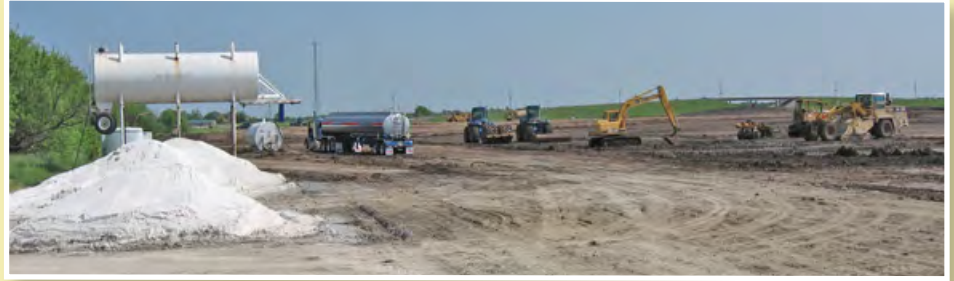
Tons of quicklime have been introduced to the soil in preparation for concrete work at Viega's plant site northeast of McPherson. This is a view from the construction offices looking north.
