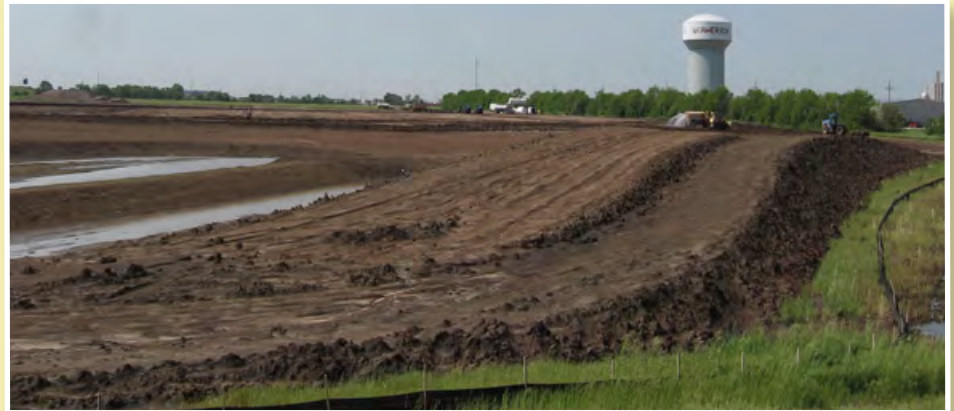
Construction crews have moved more than 202,000 cubic yards of dirt as they prepare the McPherson site for construction of Viega's 439,000 sq. ft. manufacturing and logistics facility. This is a view from the road north of the building site.
